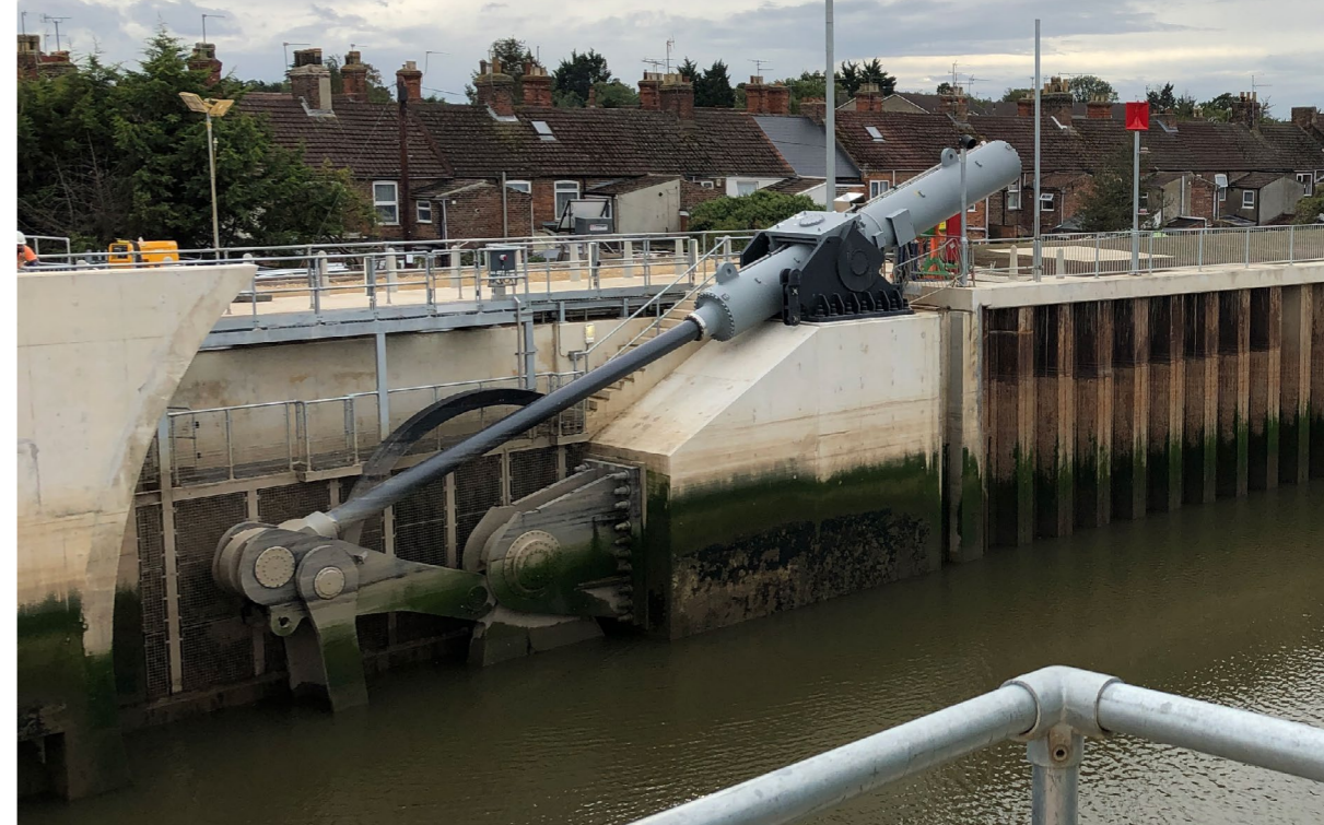
The barrier, pictured here in the open position, will bring wider social and economic benefits in addition to increased flood protection.
