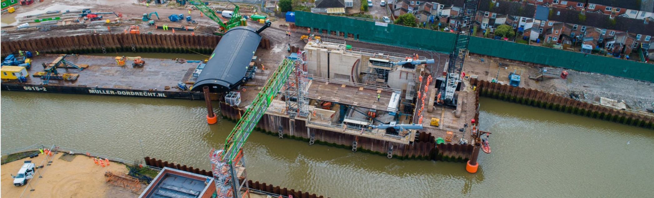
An aerial view of the construction site as the rising sector gate is unloaded from the barge that transported it from the Netherlands.
