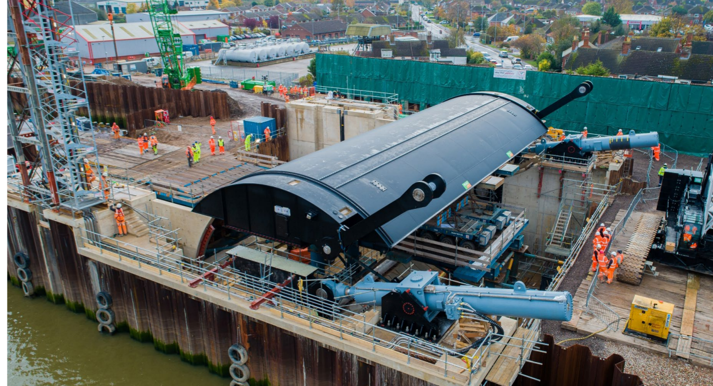
A drone image of the construction site taken during installation of the rising sector gate.
