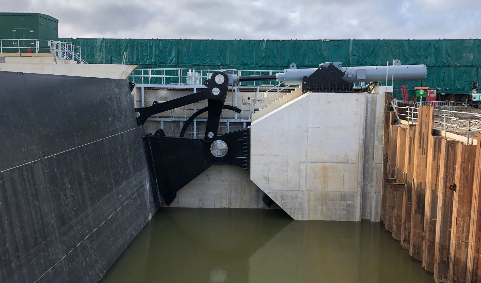
A closer view of the anchorages for the hydraulic ram and pivot on the right bank side as the gate nears the closed position during a post-installation test.
