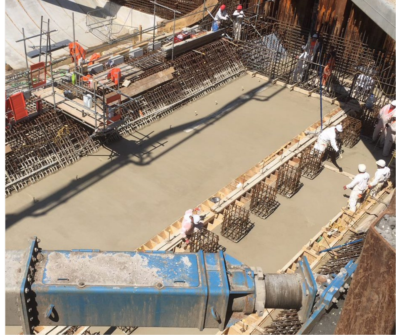
Concreting to the stilling basin. This part of the structure's base is where water falls when the gate is partially raised and is designed to dissipate the water energy before it flows downstream.
